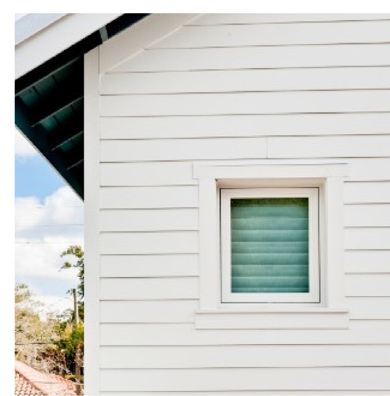
B HORIZONTAL SIDING & TRIM Material: James Hardie Cementitious Siding Color: White Dove (OC-17) Walls
